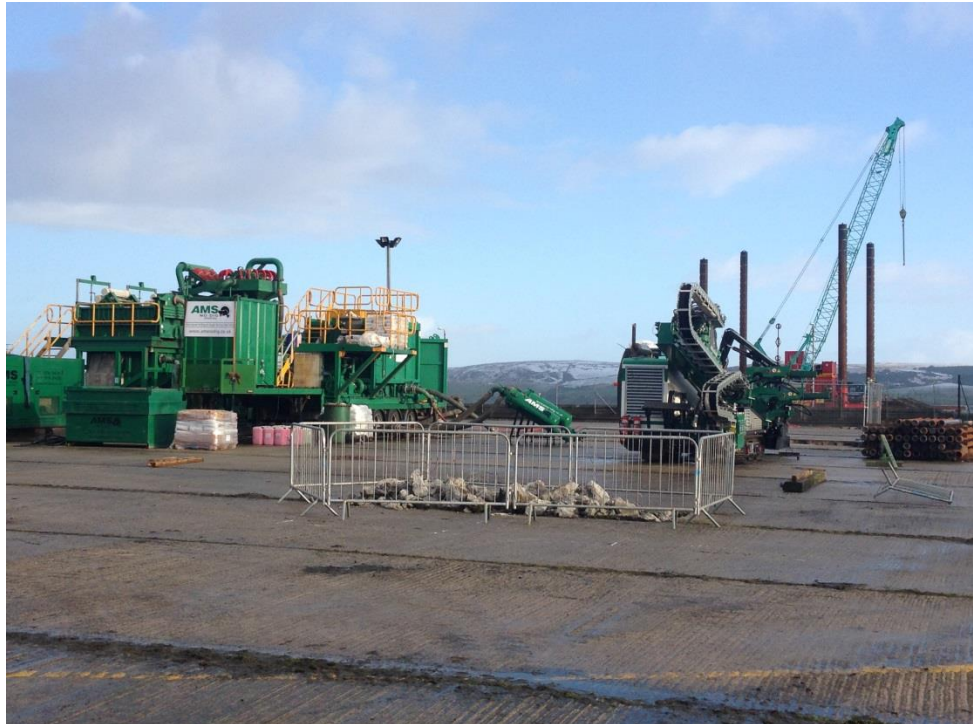
Site setup at Port Rodie including the Prime PD60/30 and mud recycling equipment
