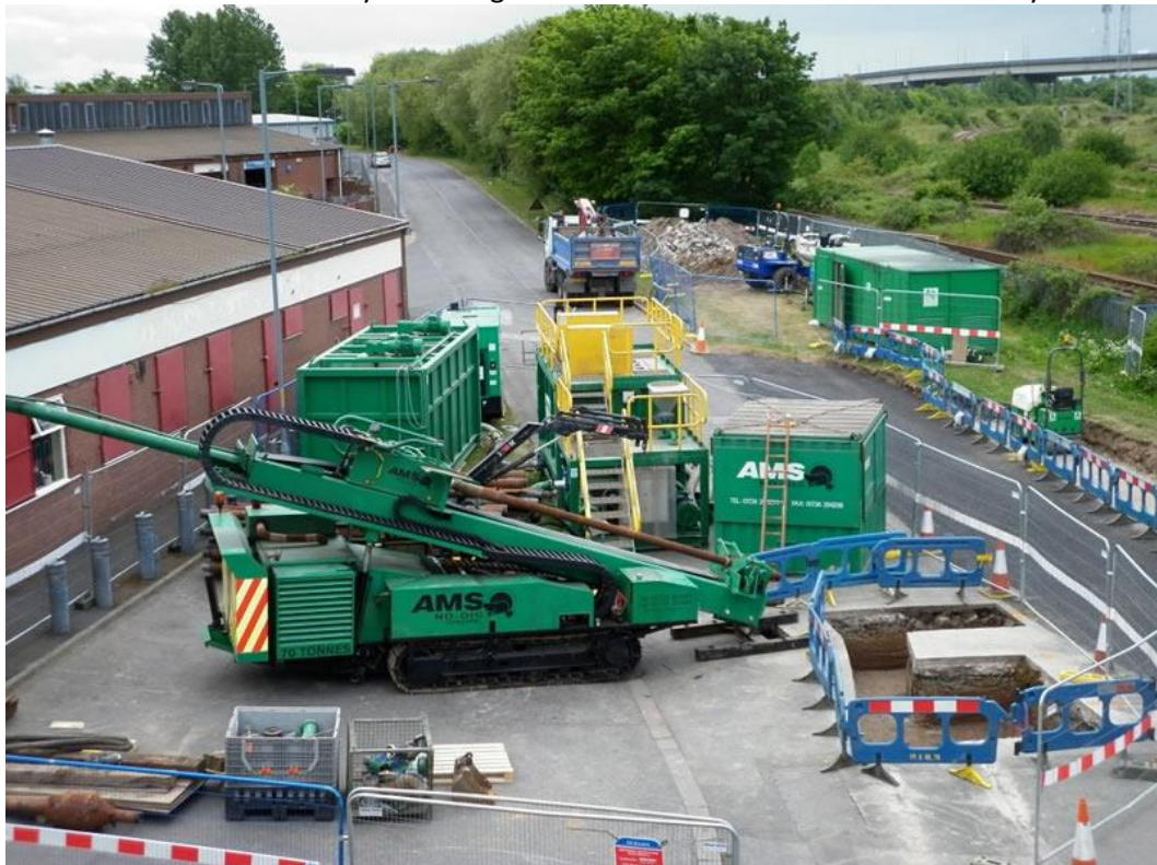
The AMS No-Dig Powerbore 70 tonne drill rig set up on site. The mud recycling system can also be seen behind the drilling rig
